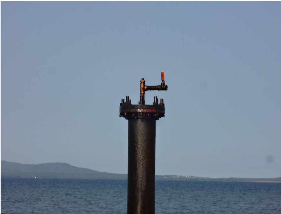
Photo 1 – Oil Leakage from Extension Pipe of Well Repair #1
