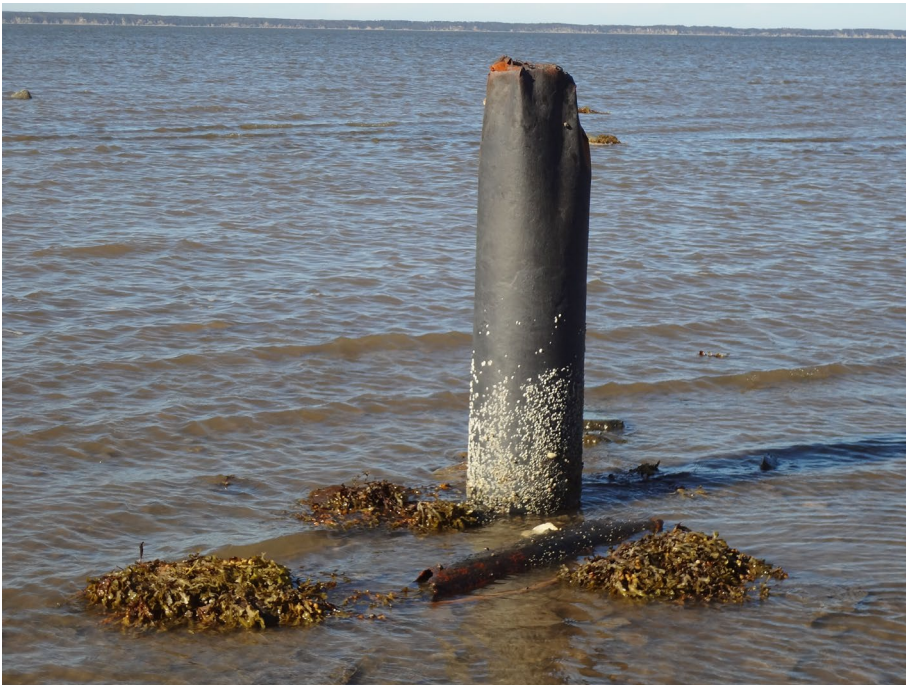
Photo 3 - Abandoned Well Casing
