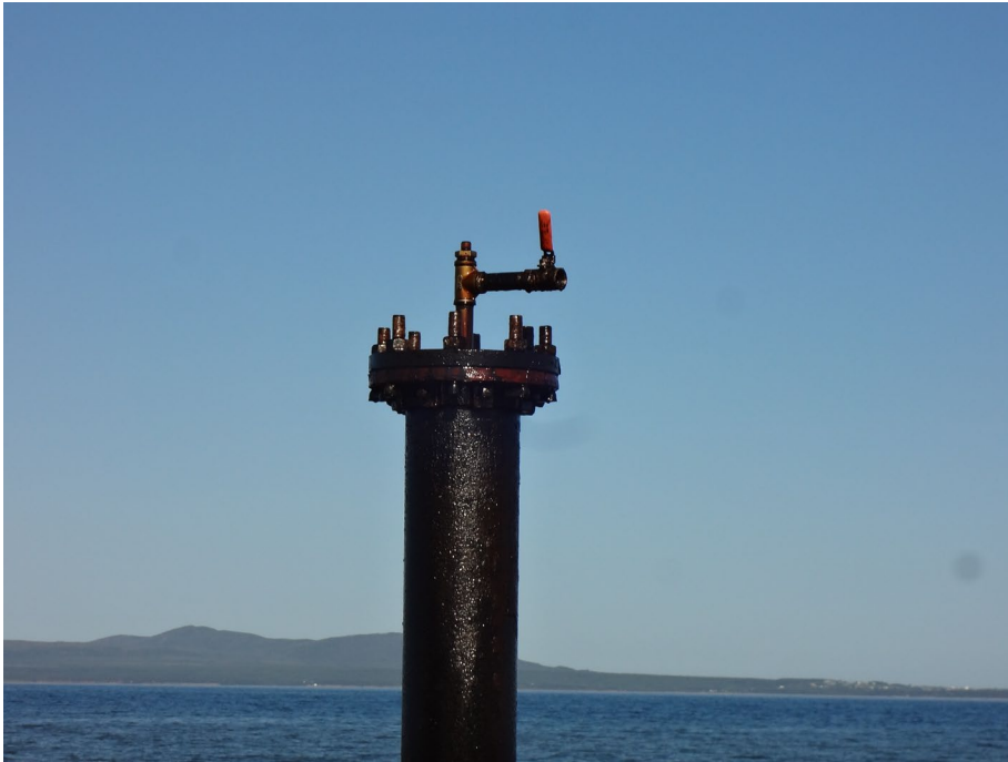
Photo 1 – Area of Observed Oil Leakage from Extension Pipe of Well Repair #1
