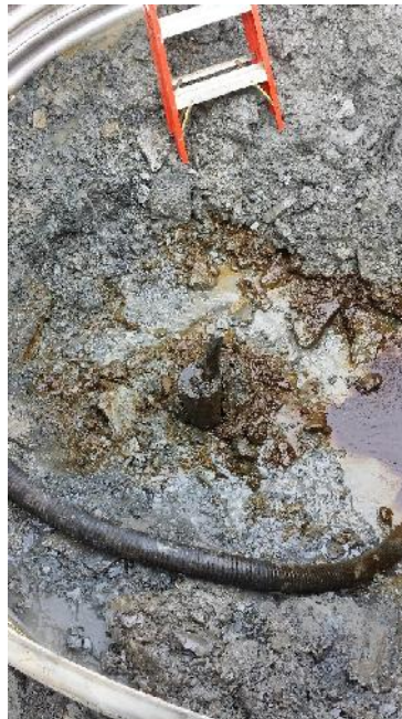
Photo 6 – Exposed abandoned leaking oil well casing No. 1.
