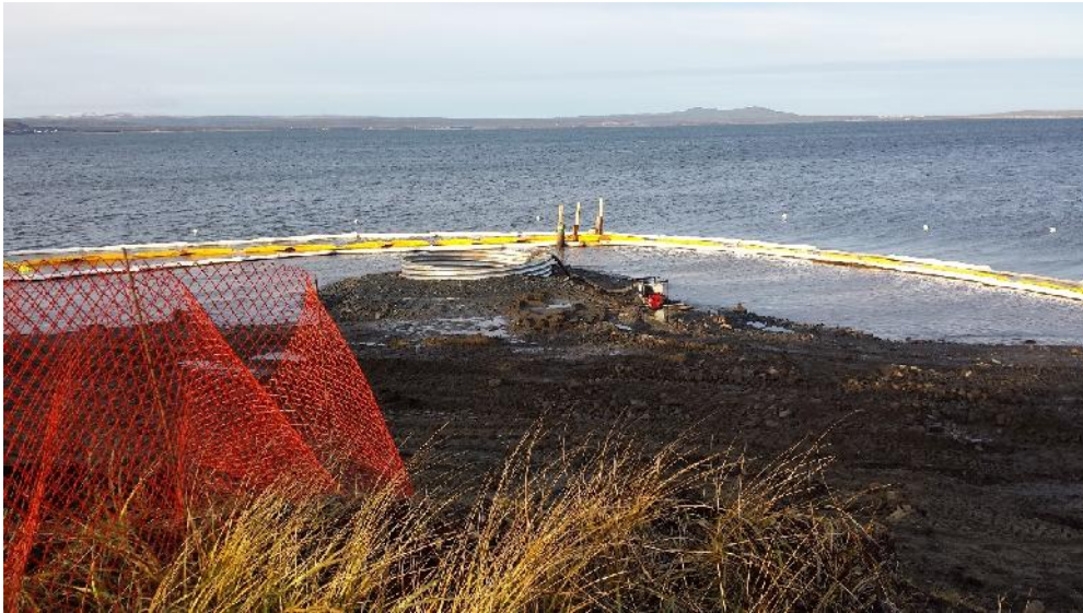
Photo 1 – View of work site at beginning of second day of construction (Well Casing No. 1).
