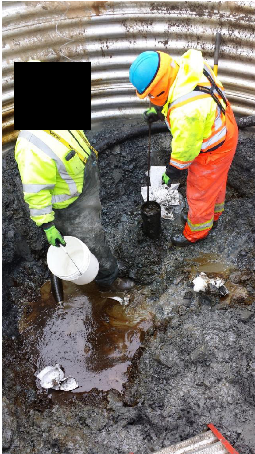
Cleaning Debris Out of Casing – Note PID Extension Hose in the Background
