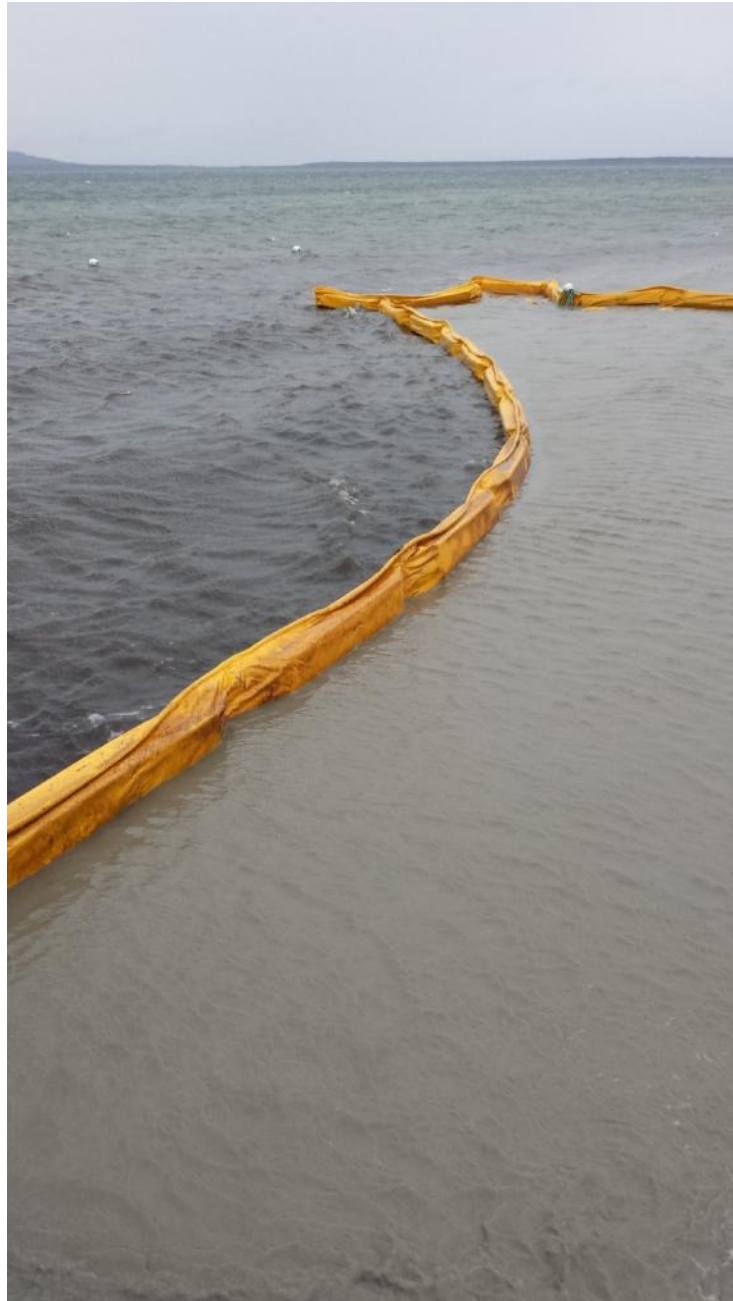
At end of Well #2 repair, the Turbidity Curtain was left in overnight to allow for settlement
