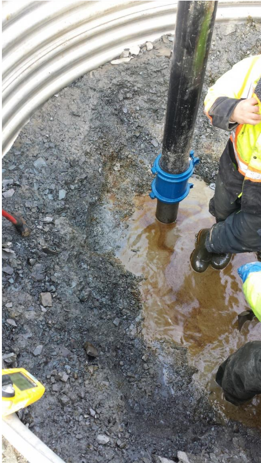
Dresser Coupling and Riser (workers had just cleaned the soil and loose bedrock down to solid bedrock. Note the oil on the water and oozing out from pockets in the rock).
