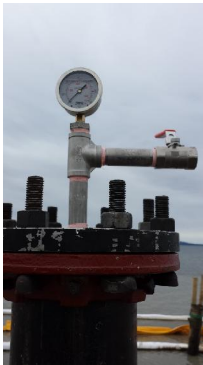
Photo 2 – View of installed pressure gauge and lockable outlet valve.
