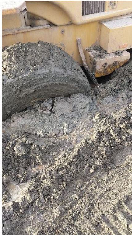
Photo 5 – Contractor encountered challenging conditions along beach access.
