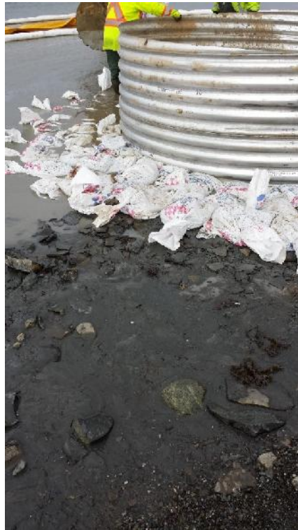
Photo 3 – Sand bags used to help seal around perimeter of 3.6 m \varnothing culvert.
