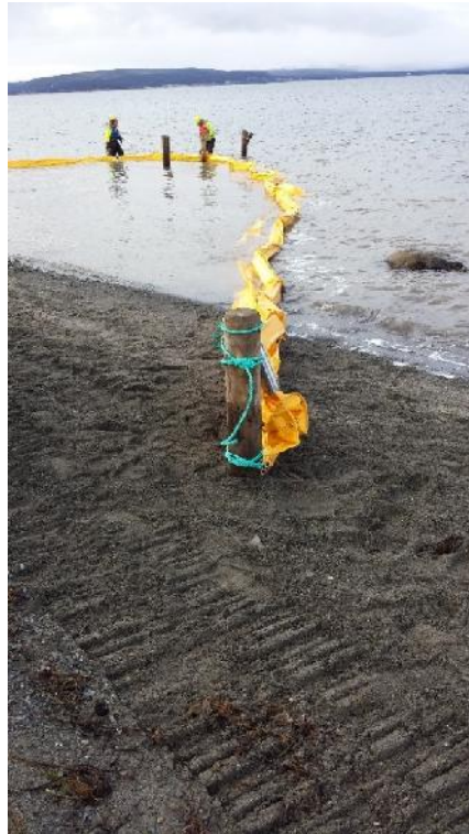
Photo 3 - Contractor installing turbidity curtain in water around well casing No. 1 work area.
