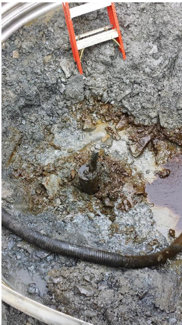
Uncovered Well Casing at about 12:30 PM.
