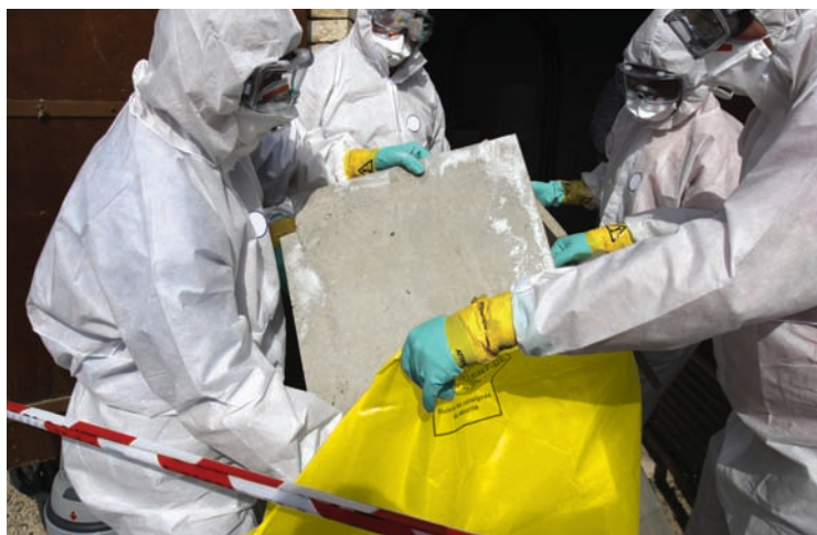
Figure 10-7 | All work involving asbestos materials must be conducted by an asbestos abatement contractor that is registered with the provincial government.
