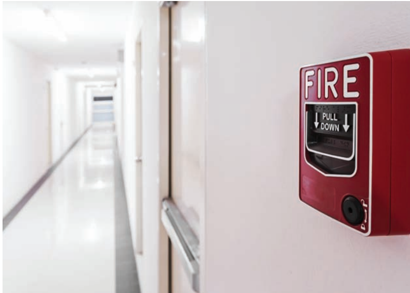
Figure 8-1 | Do you know the closest fire exit to your classroom? Do you know where the closest fire alarm is located?
