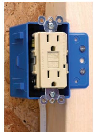
Figure 16-7 | The GFCI is designed to sense current leaks large enough to cause serious personal injury. They operate on line-to-ground fault currents.
