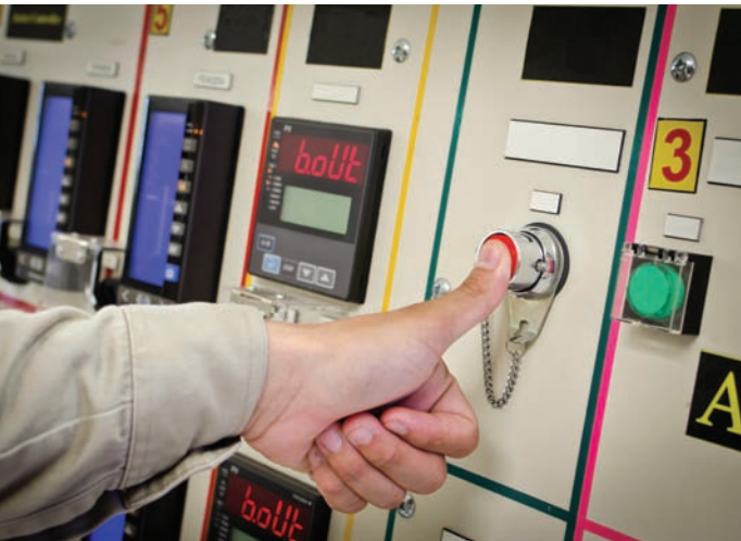
Figure 17-6 | How do the controls pictured here reflect safe work procedures?
