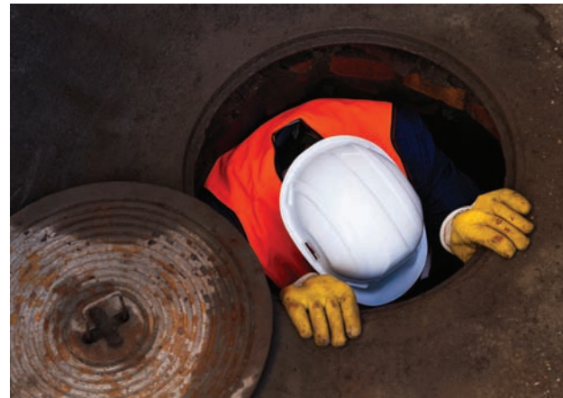
Figure 18-2 | What additional hazards could be present at this worksite?
