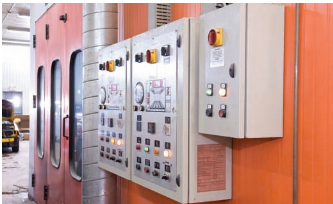
Figure 10-19 | Ventilation is a common engineering control for health hazards. It can be effective when it is designed properly for the task and is adequately maintained. These are ventilation control panels on the wall of a spray booth in an automotive shop.
