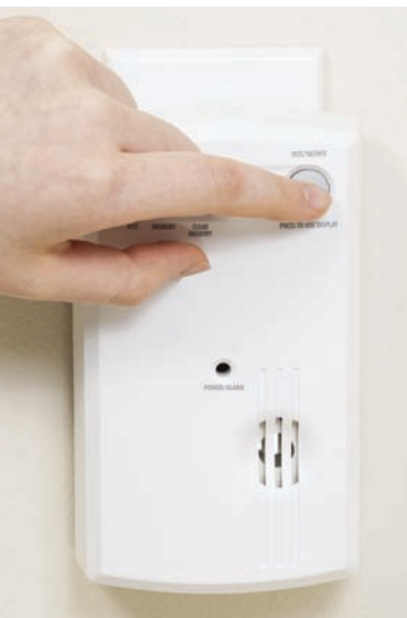
Figure 10-12 | Smoke and carbon monoxide detectors should be tested frequently to ensure they are operating properly. During the test is a good time to remind family members of what to do when alarms sound.
