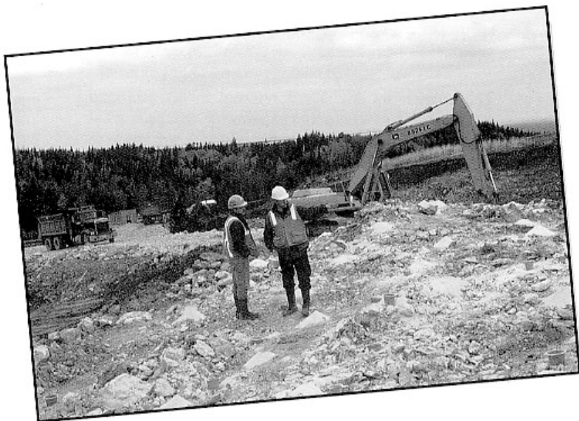
Rod Mercer (right), Project Geologist, and Rick Legge, Project Engineer, discuss the initial mining of Pennecon's barite/celestite deposit at Boswarlos.
