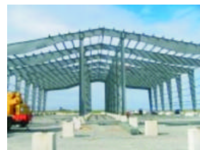
Demonstration Facility, July 2004
